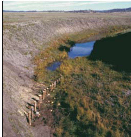
Post trimmed to 10° angle of declination from horizontal. Photo by Courtney White.
